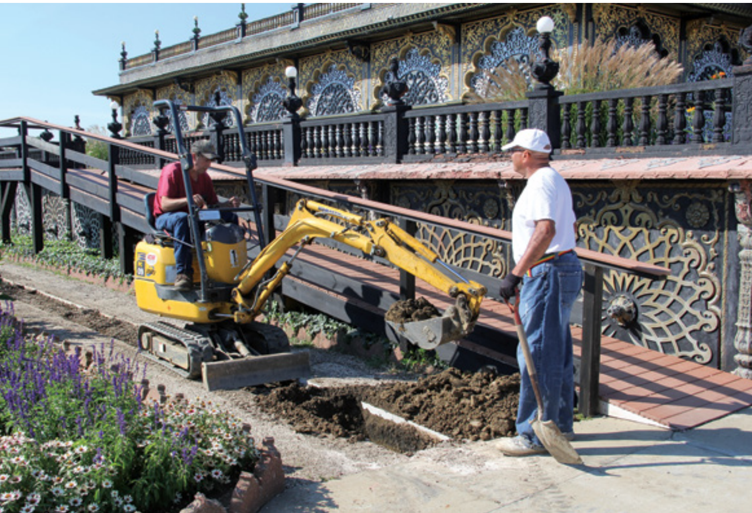
Above, a backhoe digs a trench for a drainage pipe, being laid at right.
